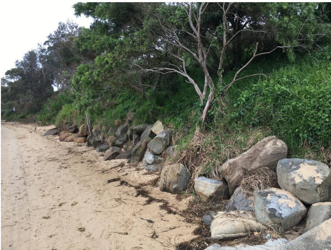
Figure 2.15 Uncertified Rock Seawall in Zone 3A
