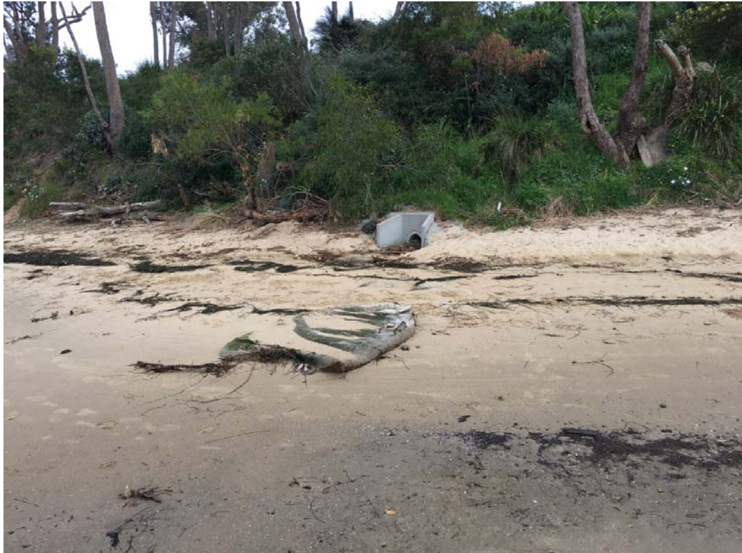
Figure 2.13 Stormwater Outlet and Damaged Geotextile Bag at Chainage 535 m
