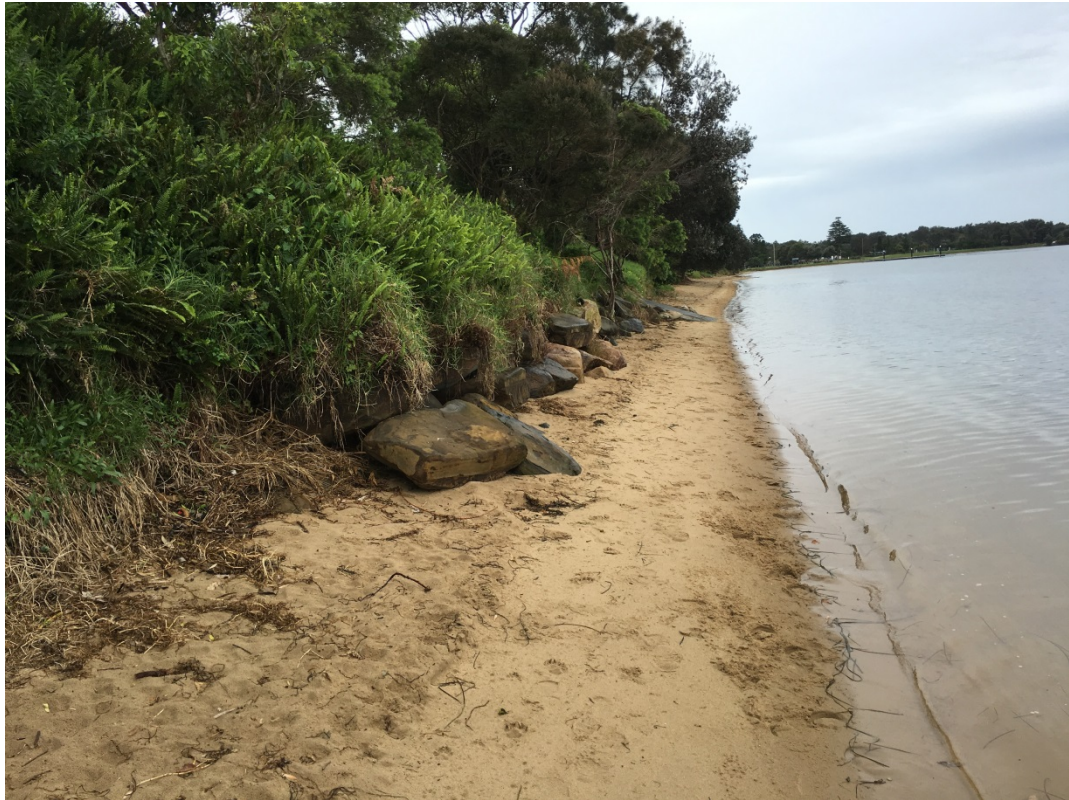
Figure 2.16 Uncertified Rock Seawall in Zone 3A
