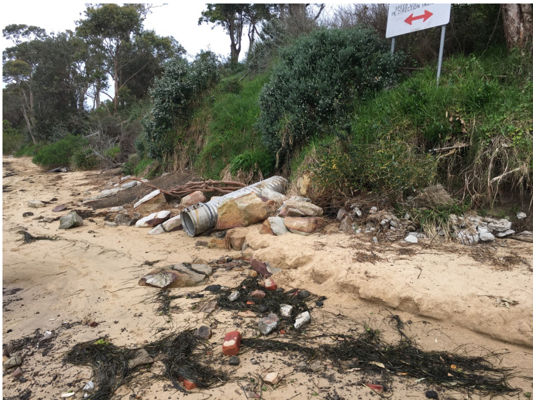
Figure 2.14 Stormwater Outlet and Rubble Debris at Chainage 590 m
