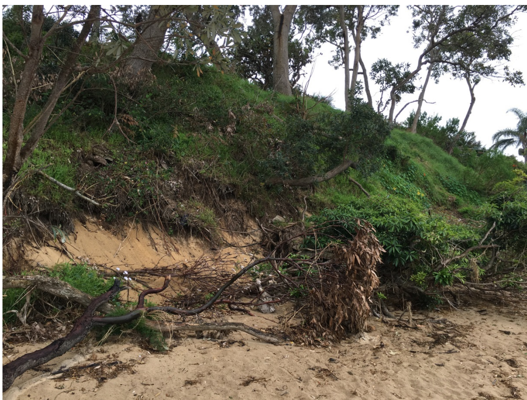
Figure 2.10 Back Beach Embankment in Zone 2B with extensive land-slip (~Chainage 550 m)
