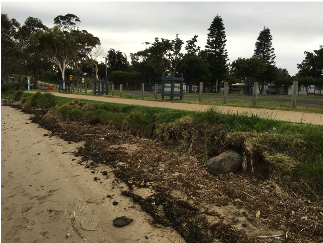
Figure 2.23 Minor Erosion, Typical of Chainage 990 m to 1040 m
